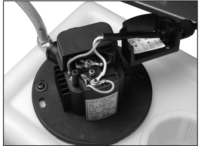
Figure 44. Pump junction box.
