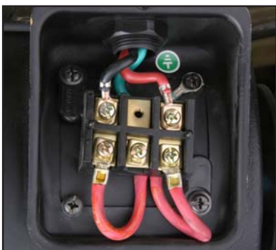
5HP 1-PHASE 220V MOTOR
