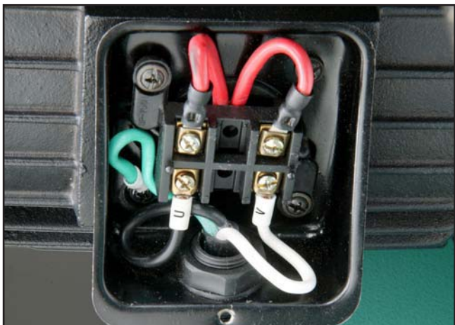
Figure 91. Motor junction box wiring.
