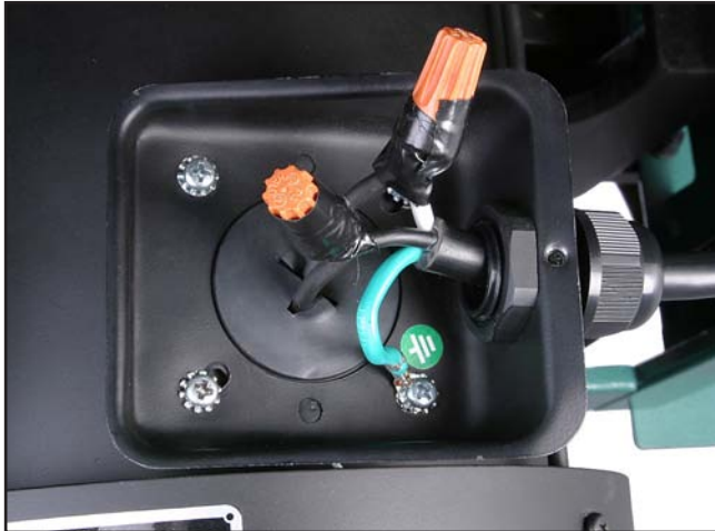
Figure 154. G0605X1/G0696X motor junction box.
