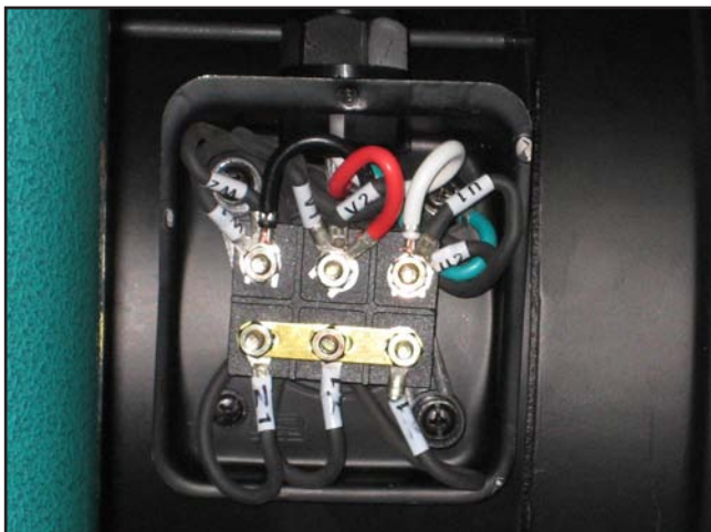
Figure 156. G0606X1/G0697X motor junction box.
