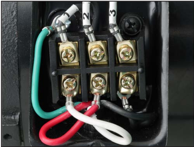
Figure 53. Motor junction box wiring.
