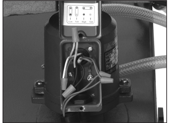
Figure 51. Pump motor wiring.
