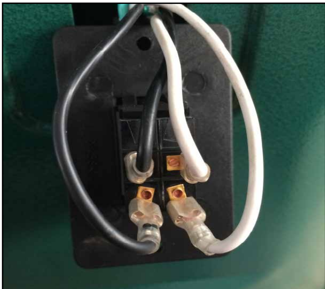
Figure 28. T26418 switch connection.
