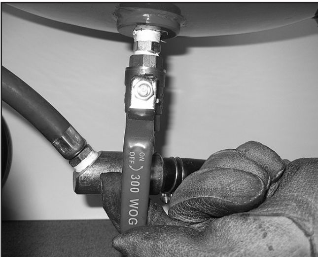
Figure 14. Sand metering valve in the full-open position.
