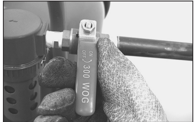
Figure 8. Tank air supply valve, closed.
