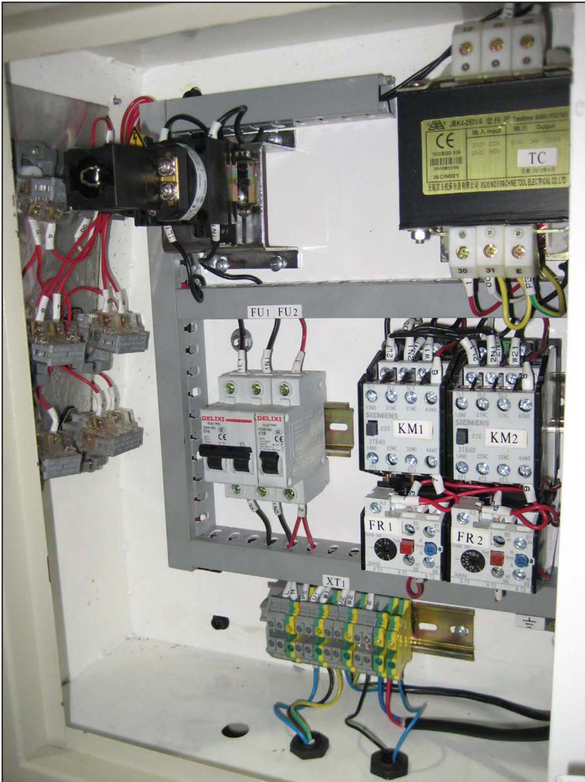
Figure 50. Electrical panel and control panel wiring.
