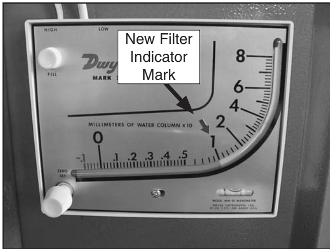
Figure 19. New filter installation mark example.
