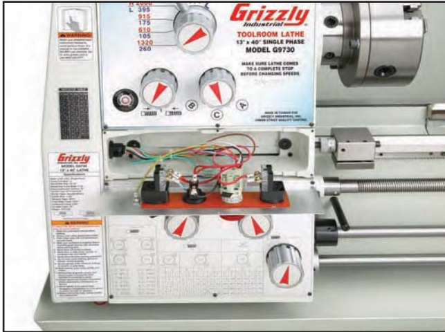
Figure 146. Control panel wiring.
