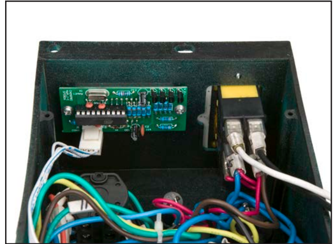
Figure 96. Control panel wiring (top).
