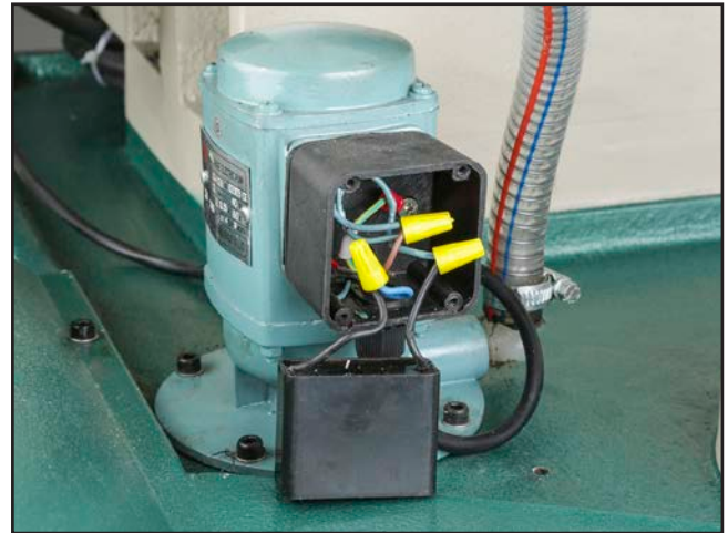
Figure 87. Coolant pump wiring.
