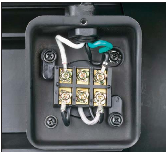
Figure 66. Bandsaw motor wiring.
