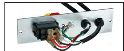
Figure 97. G1014Z switch wiring.
