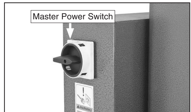
Figure 11. Master power switch.
