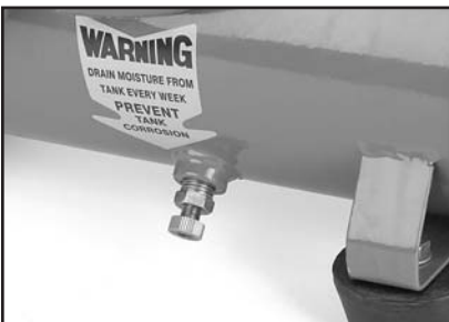
Figure 10. Tank drain valve.
