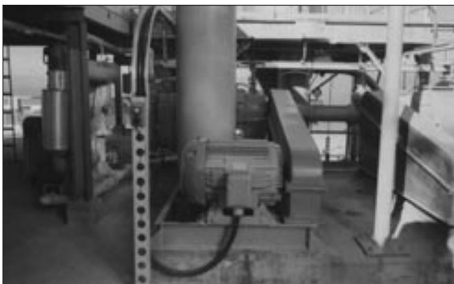
Control Cable Entering Pushbutton and Power Cable Entering Motor Terminal Box from 6 Inch Channel Cable Tray System (Bottom entries provide drip loops to prevent moisture flow into enclosures.)
